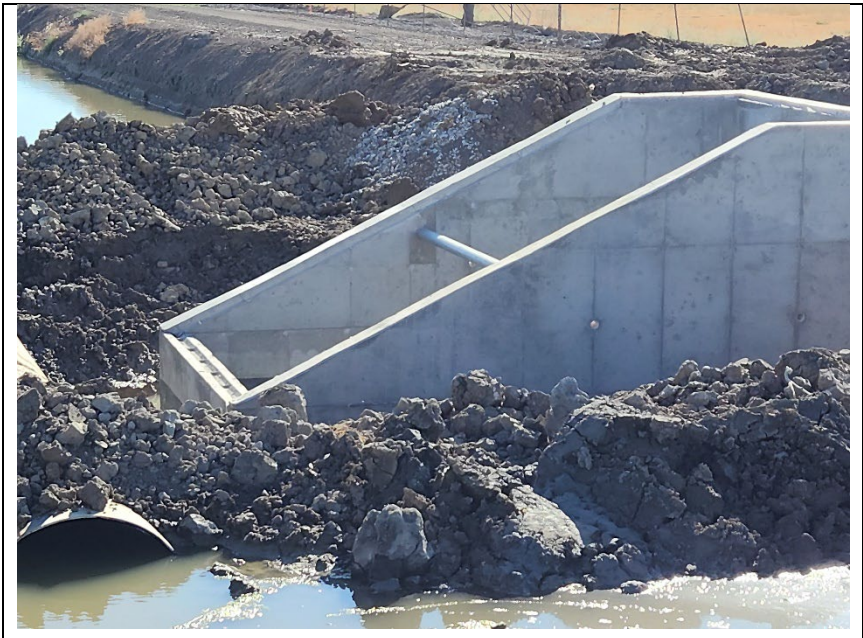
Basin Feed Pump Station inlet structure.
